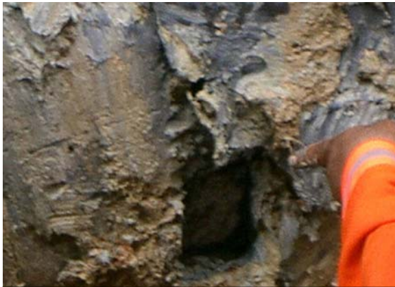
Figure 12 Coating Defect at Joint
