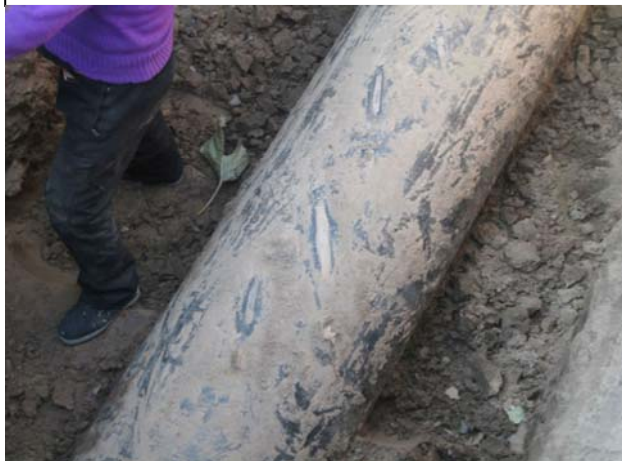
Figure 17 Multiple Coating Defects
