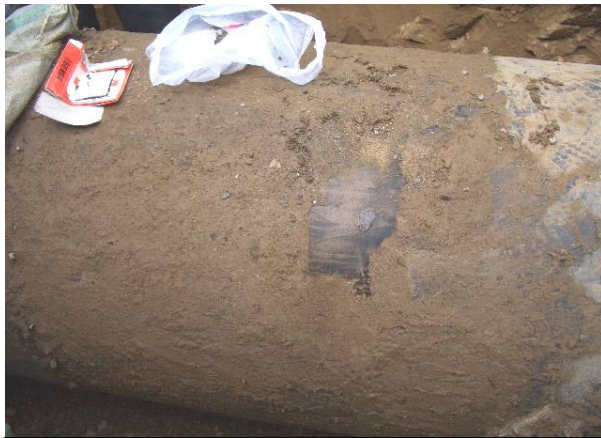
Figure 15 Coating Miss-out at Joint
